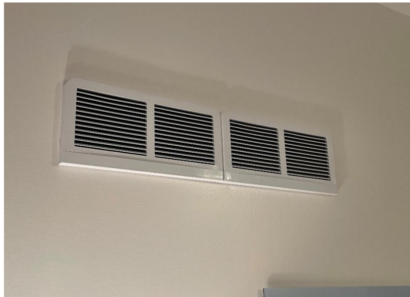
Figure 3: Impeccable Air Return Registers
